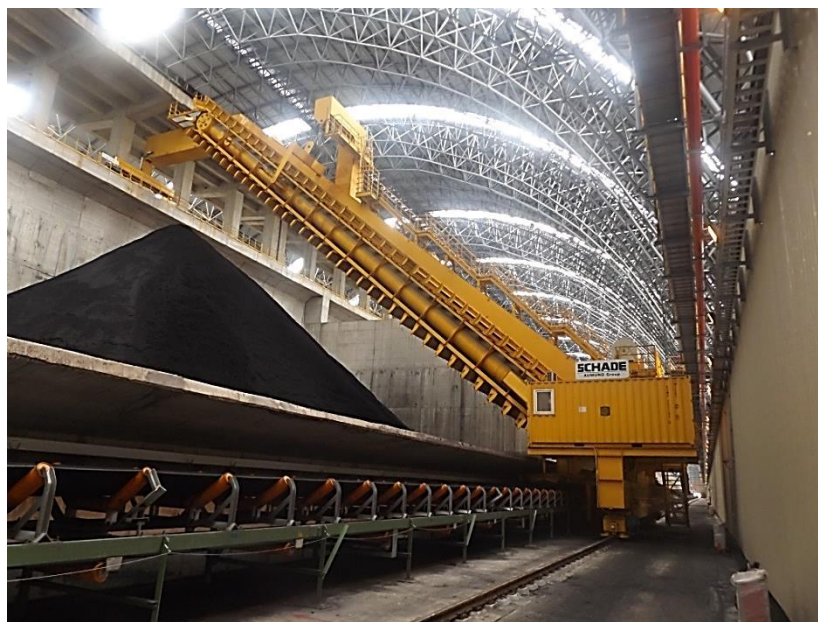
SCHADE Semi-Portal Reclaimer in operation at Ha Tinh Steel, Vietnam (example, photo SCHADE)
