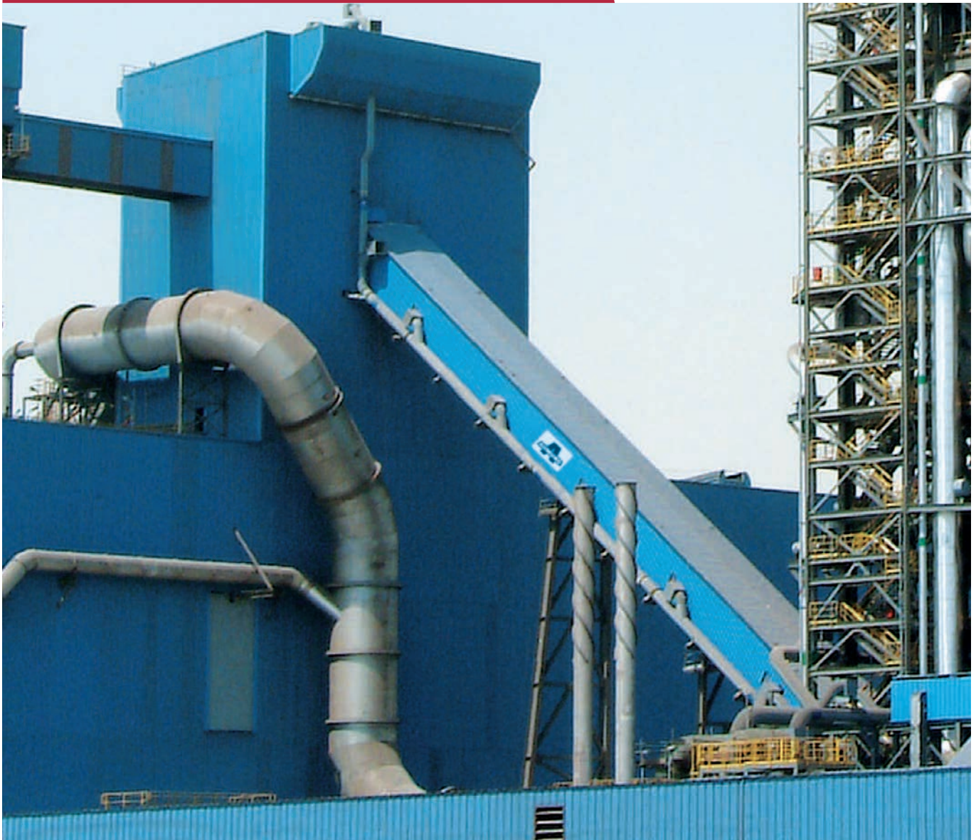
Energy efficient conveying of DRI
