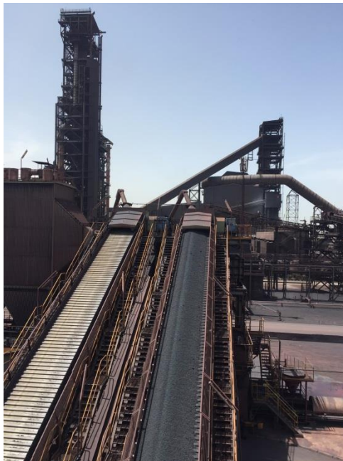
Pellet Cooling and Transport (photo AUMUND)
